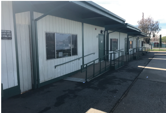
Evidence of ponding water at AC paving at portable buildings.
