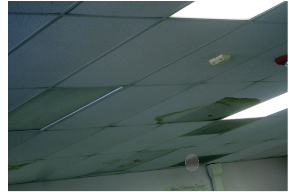
Significant water damage at ceiling tiles.
