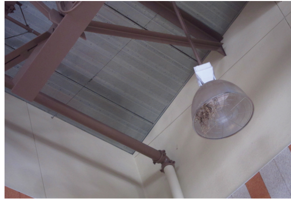
Evidene of bird roosting in Gymnasium.
