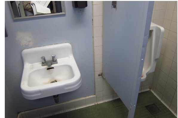
Non-accessible student restroom.
