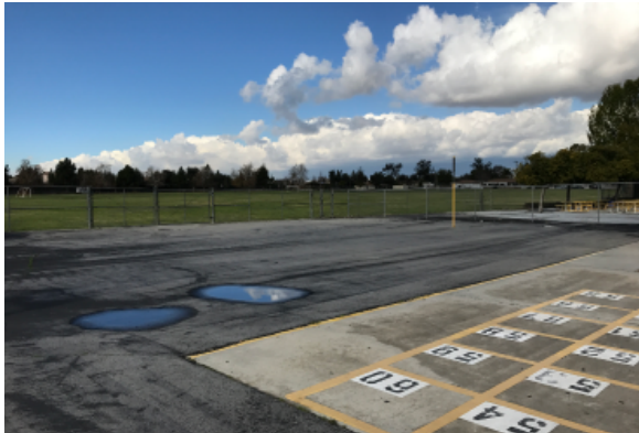
Hard courts with ponding water on asphalt and play fields.
