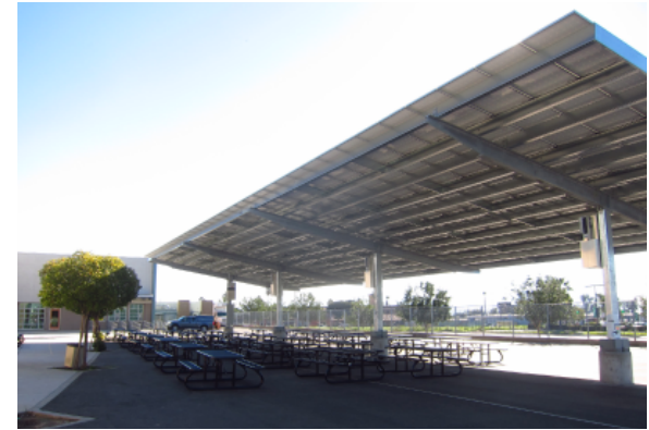
Newly installed solar photovoltaic shelter.
