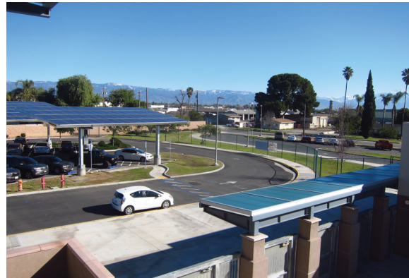
Bus drop-off area and photovoltaic shade structures in side parking lot.
