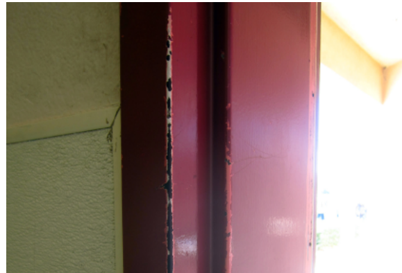
Paint deterioration at door frames with heavy traffic.
