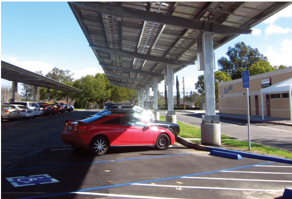
Accessible parking and photovoltaic shelter.
