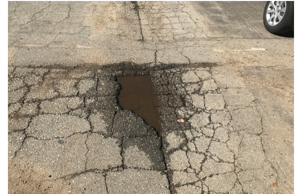
Significant damage to AC paving.
