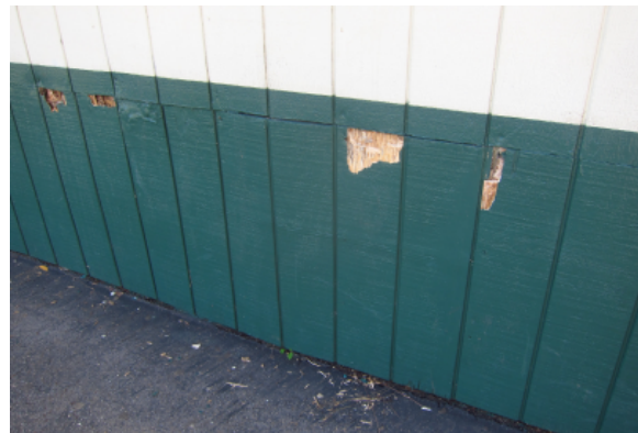
Example of damaged wood siding at modular building.
