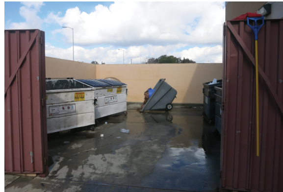
Outdoor trash enclosure with ponding water.
