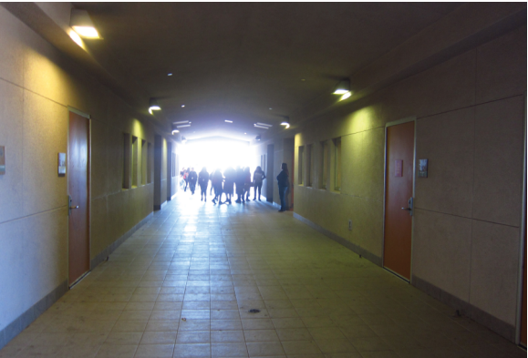
Relatively low lighting at and visual glare at the end of exterior corridors.
