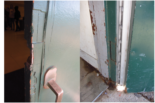
Examples of severely damaged door.
