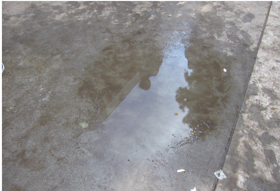
Ponding water at sunken outdoor dining court.
