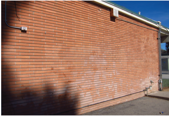
Typical brick condition.
