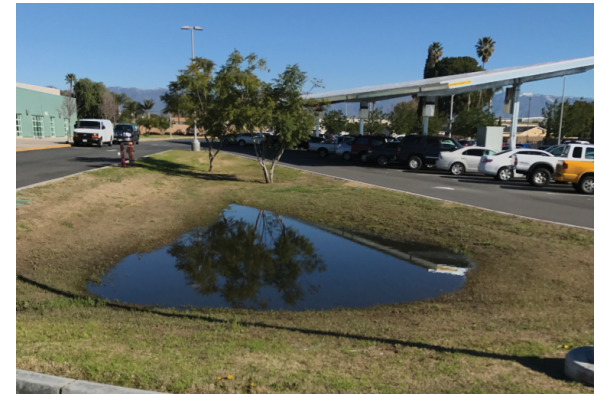
Ponding water from recent rains at front parking lot swale.
