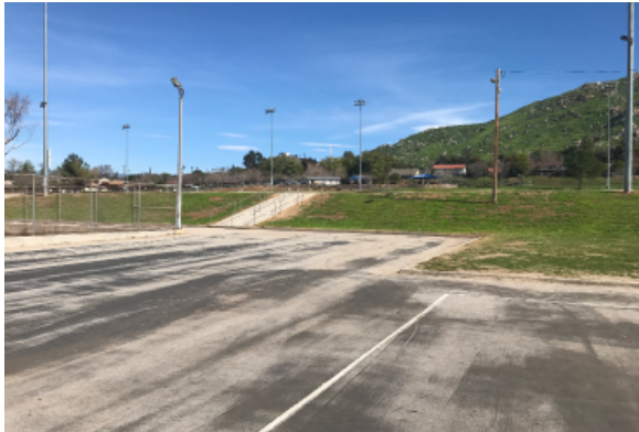
Deteriorated AC paving at hard courts.
